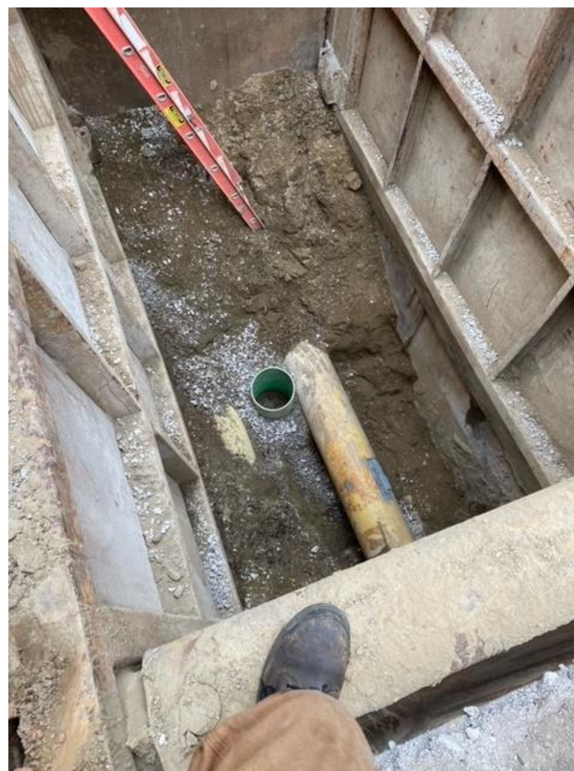
Figure 3. Chilled water pipe in question
