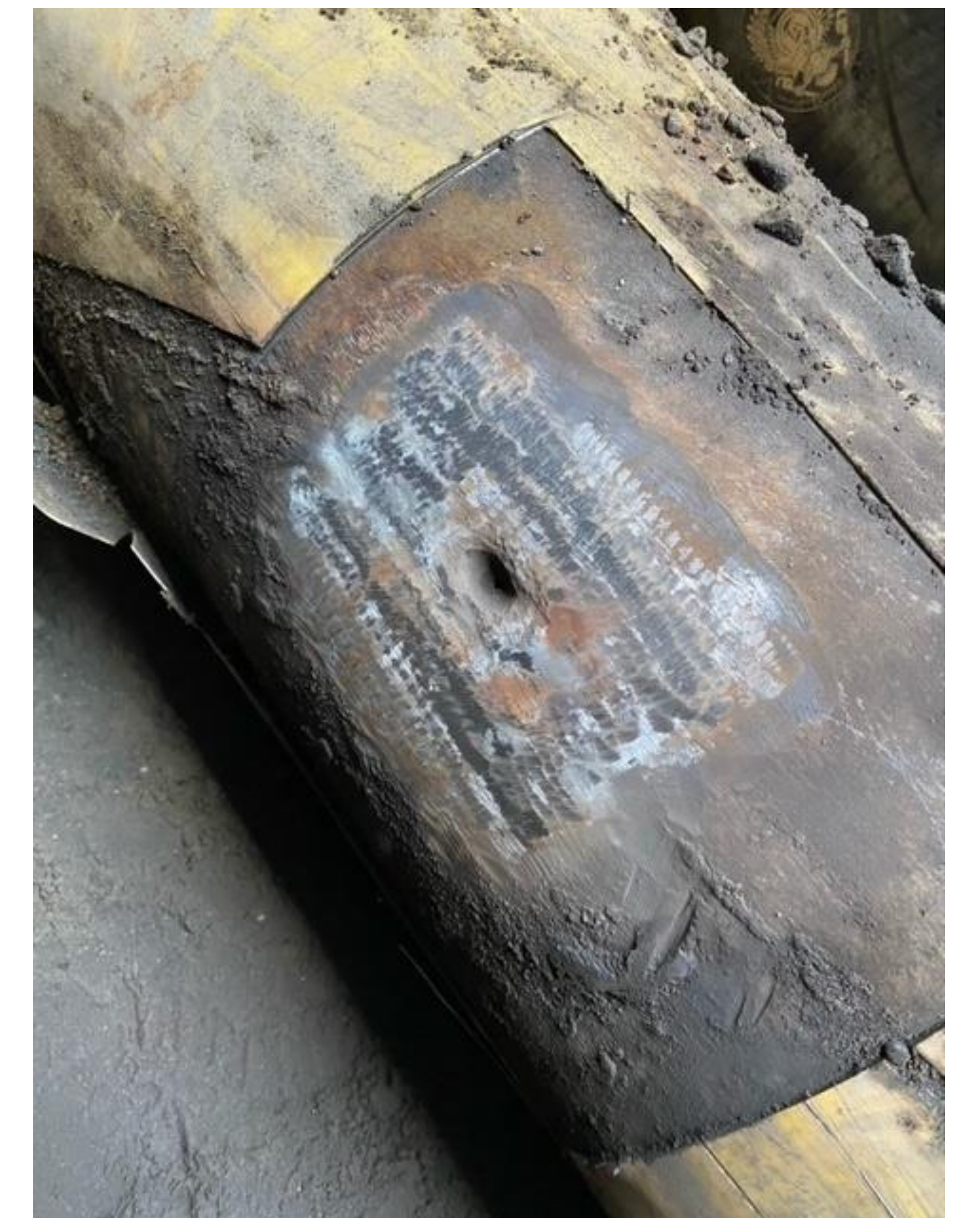
Figure 4. The hole in the pipe responsible for the leak
