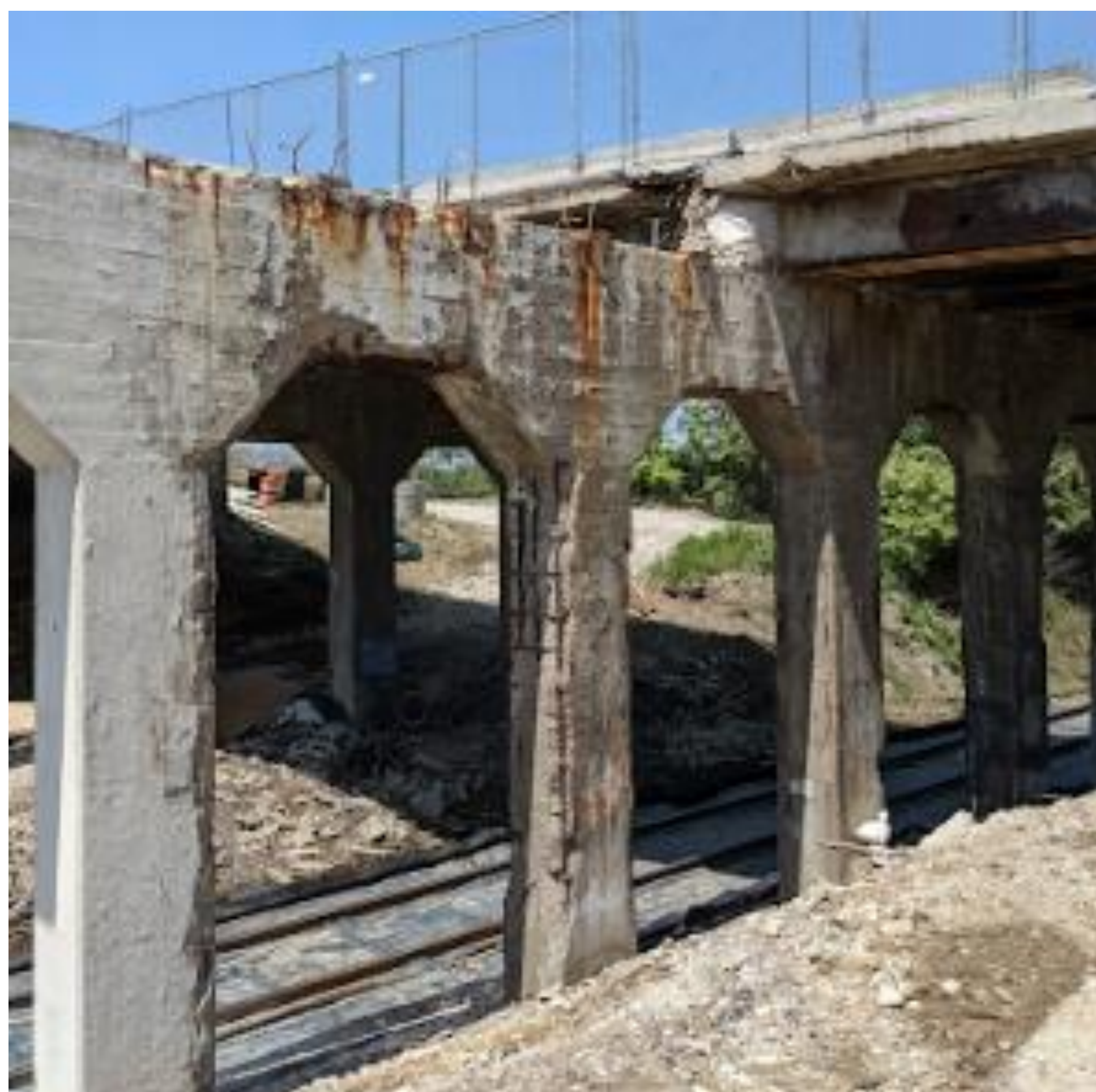
Figure 1. Memphis Road bridge closed for safety
